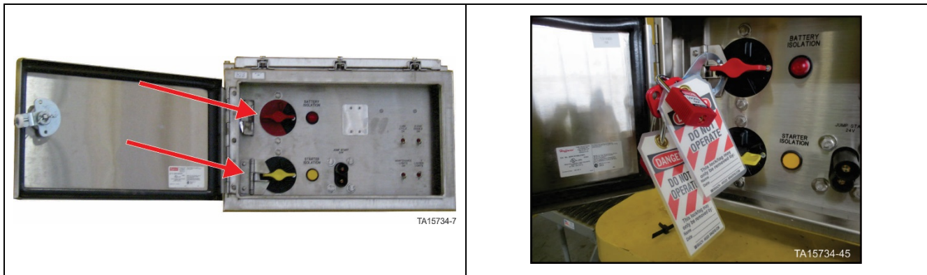
Figure 4. Battery Isolation Box – Battery isolation switch in OFF position with locks in place
